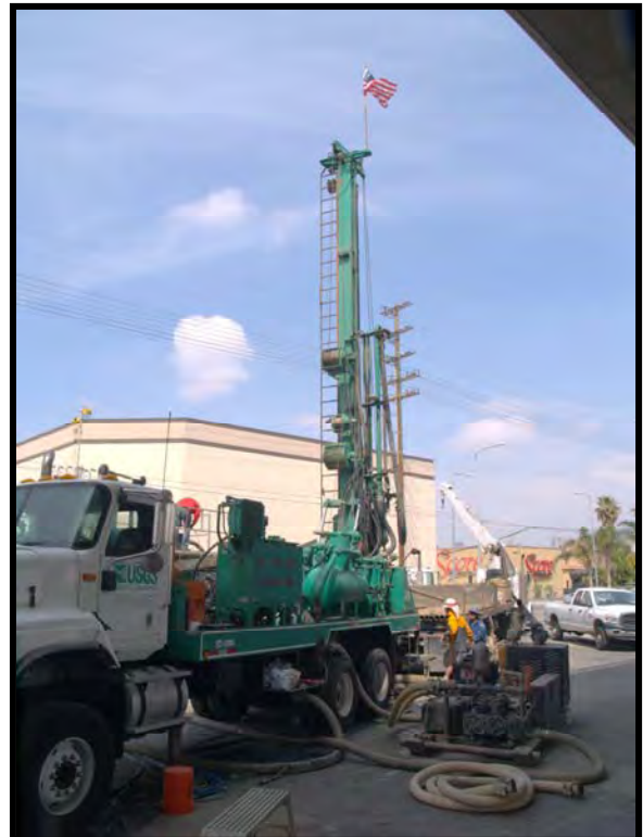
New WRD Monitoring Well LA#2
